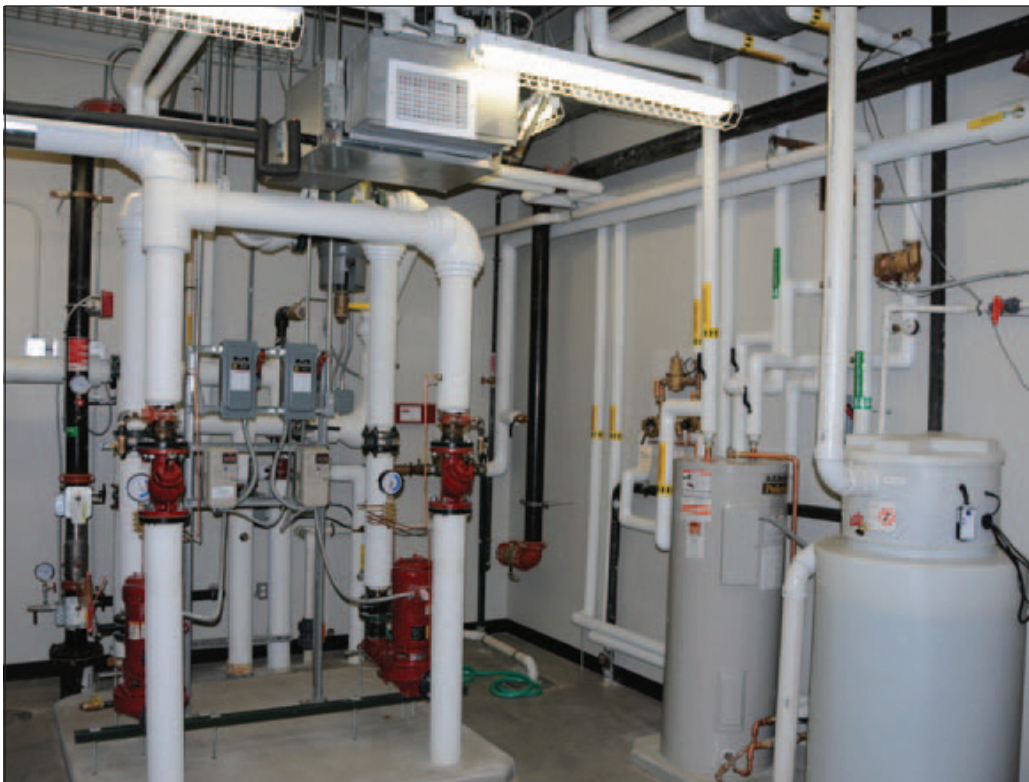
Figure 6—Interior equipment for the 21-well geothermal heat pump system in the 9,580 ft 2 (891 m 2 ) SunChips® Business Incubator, Greensburg, Kansas. From Low-temperature geothermal resources (DOE, 2010b).
